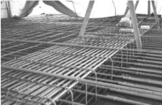
Fig. 2.3—GFRP bars used in a winery in British Columbia in 1998.
